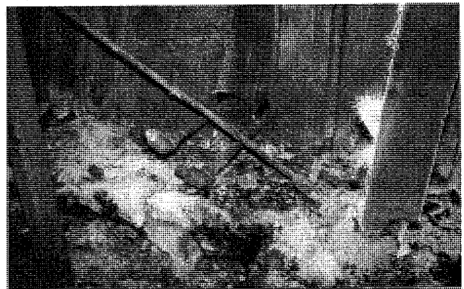
Welders working on these elbows accidentally ignited combustible materials inside the wall at this location.
