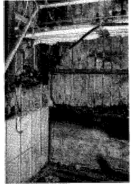
Walls in the corner of the cooler, near the mechanical room. Wallboard and plywood covered the wall at left.
