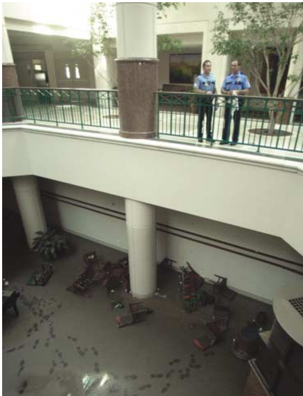
Houston police officers look over the ruined commons at the closed Memorial Hermann Hospital in Houston June 11, 2001. The hospital was forced to close after flooding damaged the building's electrical system.
