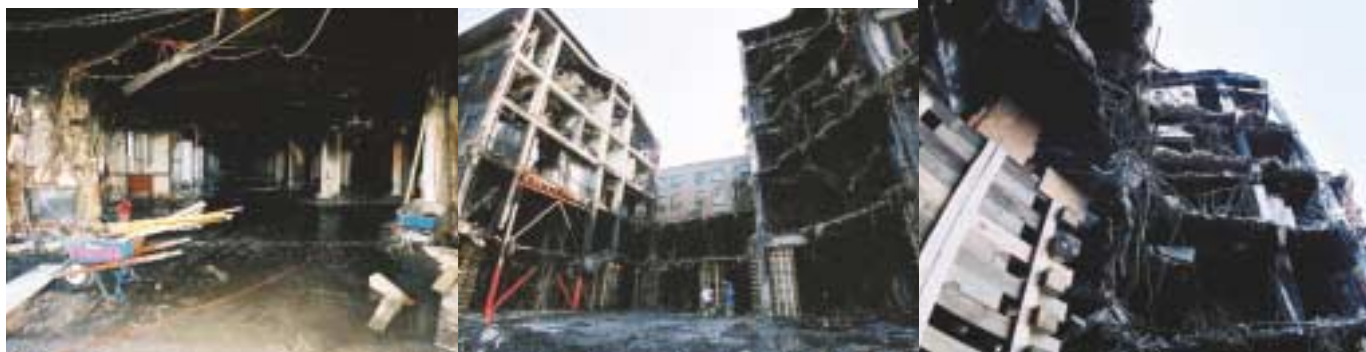
Work continues at the Pentagon attack site. The interior and exterior of the building are shown after the areas were stabilized by shoring structures.
