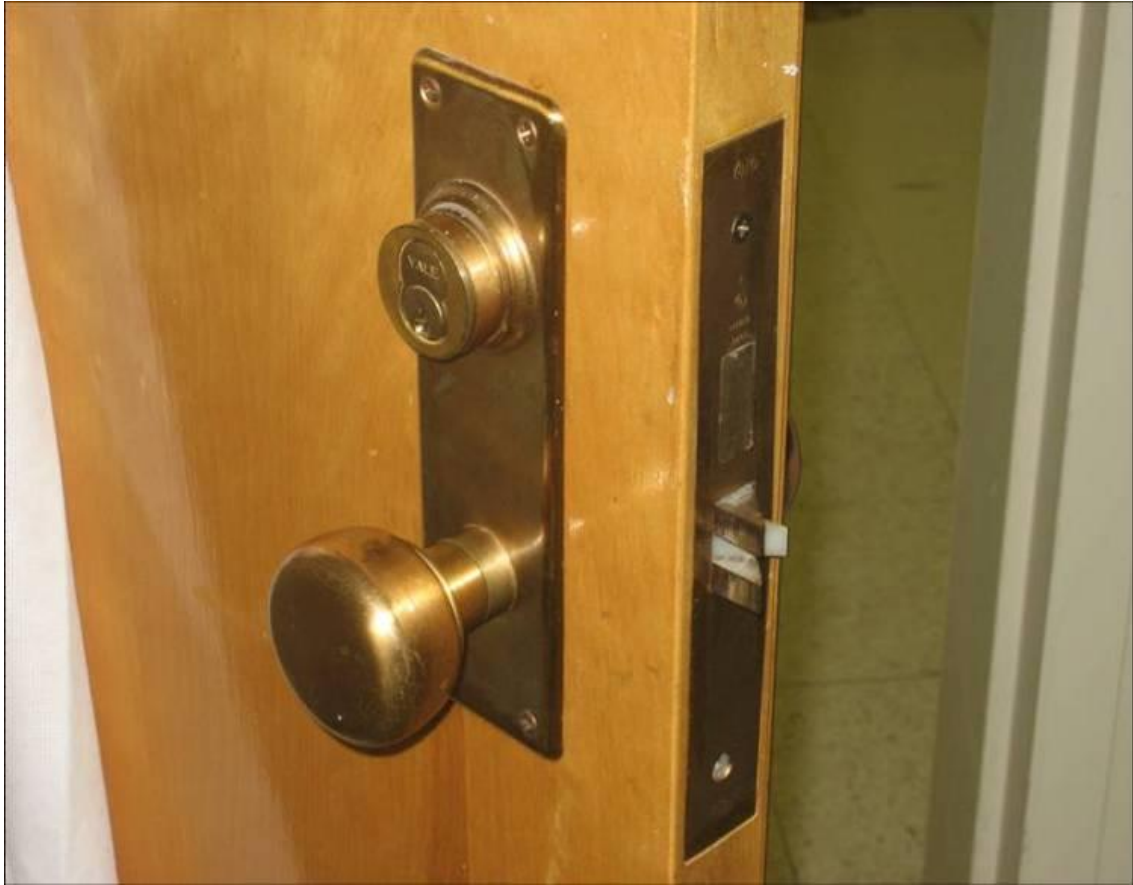
Figure 1. Door Requiring Two Operations
