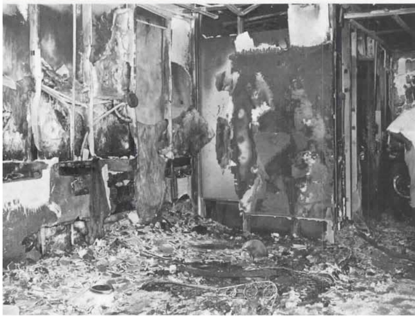
The room of origin received heavy damage. Here the bedsprings can be seen in the foreground.
