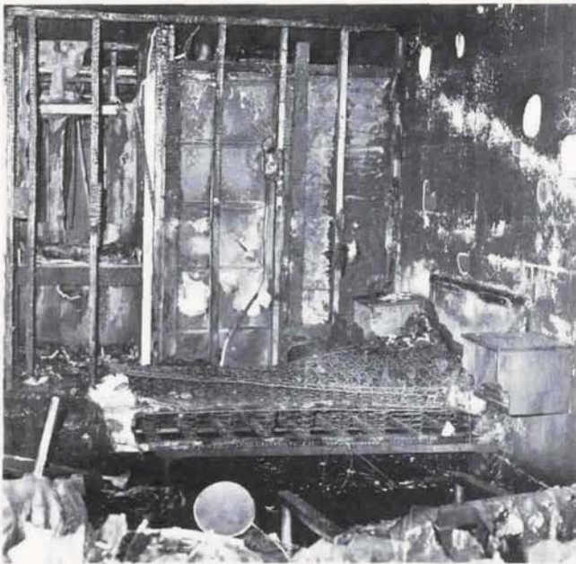
The room where the fire started. PHOTO-GRAPHIC
