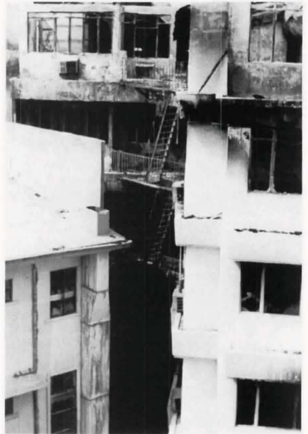
The exterior fire escape of the Hotel Filipinas as seen from the Hotel Aurelio.
