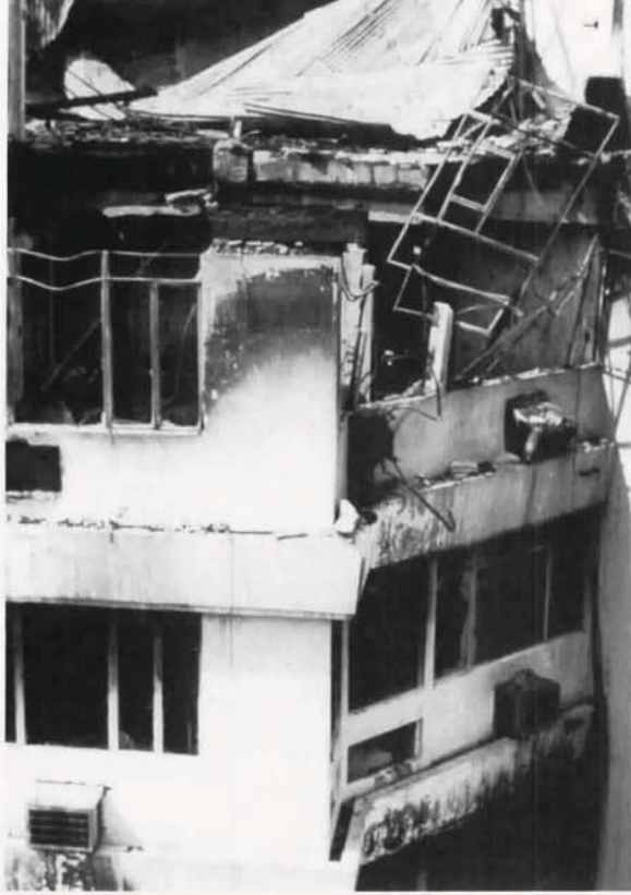
Destruction in the front portion of Main 1 building as seen from the roof of the adjacent Hotel Aurelio.
