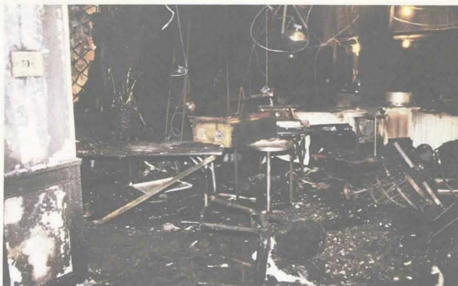
The fire originated at a propane gas grill in the function room's buffet area which had been set up near the room's main entrance.
