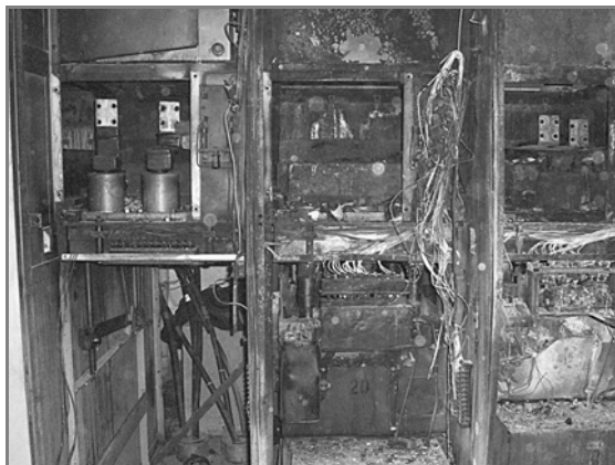
Figure L.5(c) Intense Heat Burned the Ceramic in the Arc Extinguishers. (Courtesy of Shermco Industries, Inc.)
