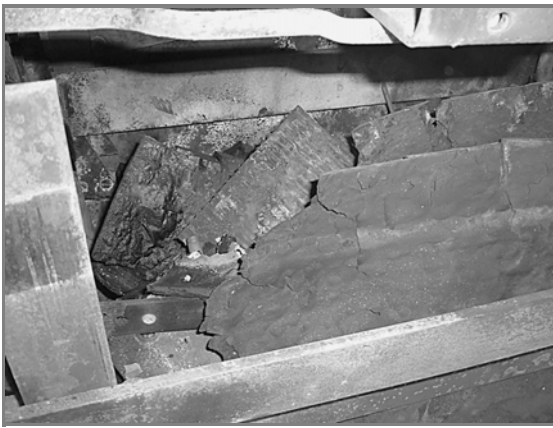
Figure L.5(d) All Bus Terminations and Insulation Was Were Destroyed. (Courtesy of Sermco Industries, Inc.)
