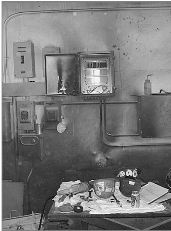
Figure L.5(b) All Six Circuit Breakers and Their Enclosures Were Destroyed. (Courtesy of Shermco Industries, Inc.)
