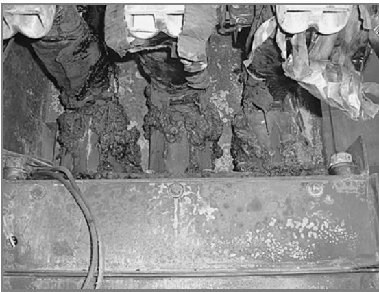
Figure L.5(e) All Metal Inside the Circuit Breaker Was Vaporized or Melted. (Courtesy of Sermco Industries, Inc.)
